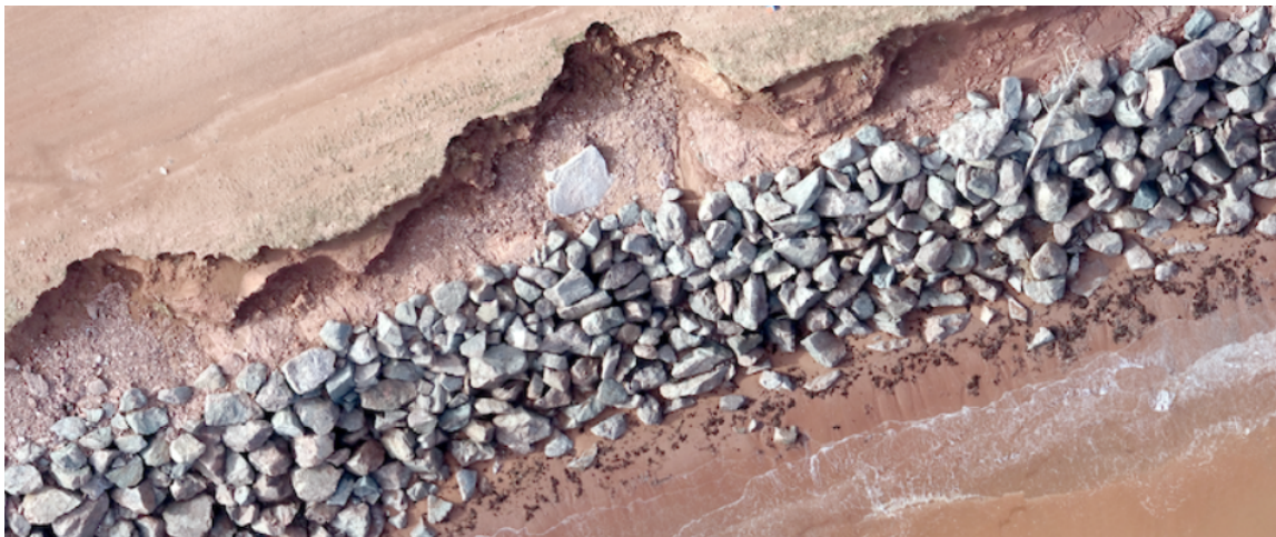
Figure 10 – Example of overtopping erosion at armourestone revetment. Source: UPEI
